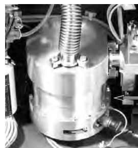
LDS valve (connected to the TMP rear)
